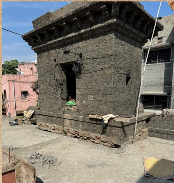
DAMEGE AT THE BOTTEN OF STRUCTURE SO TO BE REPAIR
