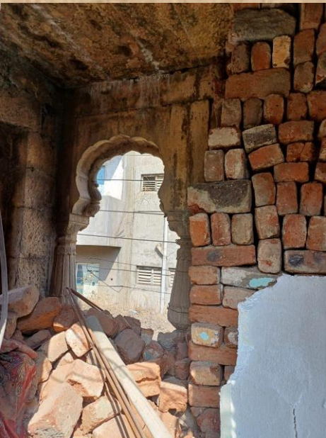
EXTRA MATERIAL SHOULD REMOVE AND SHOUD GIVE PROPER FINIDHING FROM INSIDE
