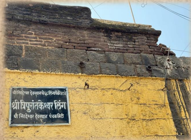
DETORINATION OF STRUCTURE IS STARTED SO TO BE REPAIRED
