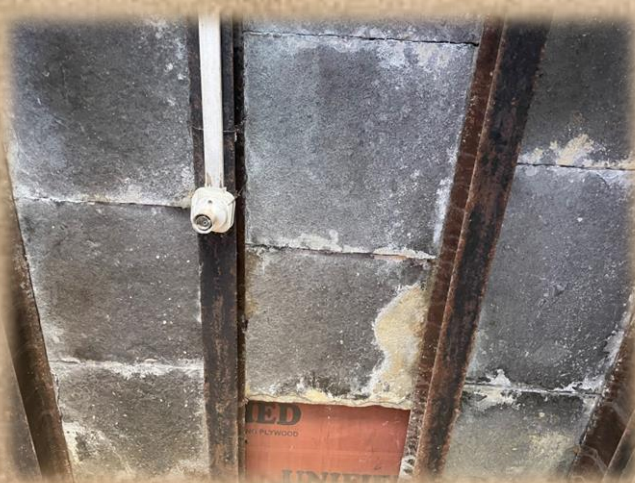
JOINTS IN THE CEILING GET WEAK AND AT SOME PART TILES ARE MISSING SO NEED TO BE REPAIRED
