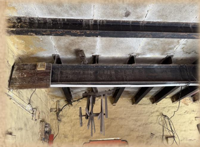
GERDER GOT OLD BY THE TIME RUSTING IS STARTED SO HAVE TO BE REPLACED OR REPAIR
